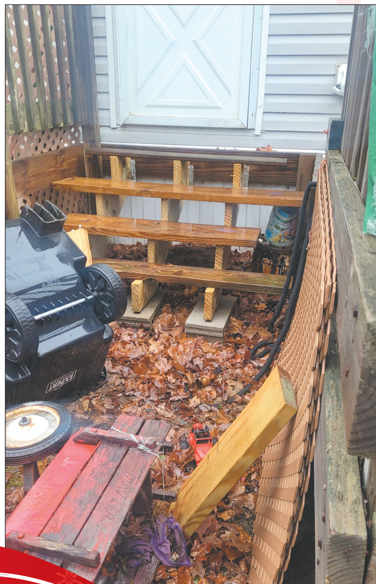
COURTESY PHOTO After her porch steps broke, Laurel Belstra said she set up a couple of cement blocks with boards over them as a substitute; as winter approached, however, she realized this couldn't be a permanent setup.
